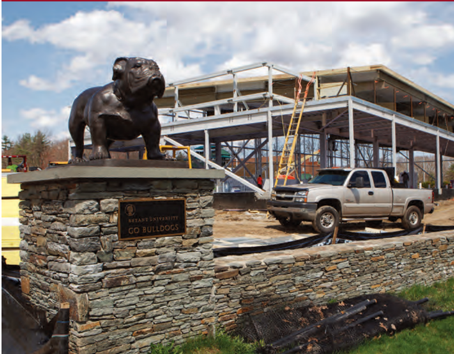
The Bryant Bulldog statues, a gift from the Class of 2009, oversee construction of the new Weight and Conditioning Center in the endzone of Bulldog Stadium.
