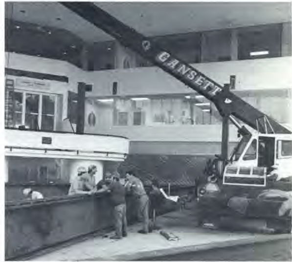
Steel I-beams had to be hoisted and swung into place, gently of course because they fit just right, inside Salmanson Dining Hall to support the new faculty office suite under construction.
