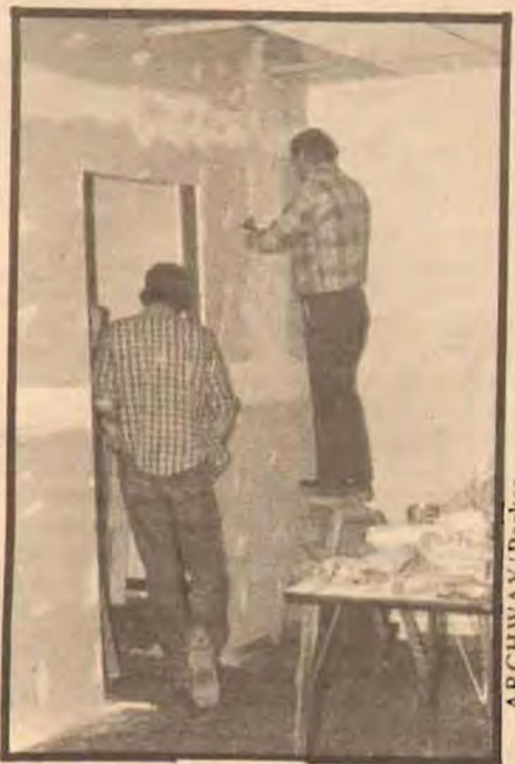
Moving In Work on the new Audiovisual Room, to be located in the former Room 277. Work is expected to be completed after Spring Break.
