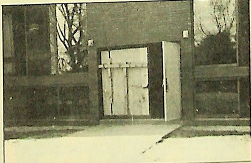
Down three window is just another example of the widespread vandalism.
